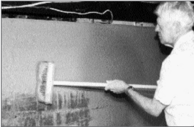
Interior Basement Application
